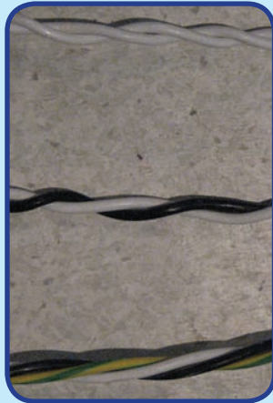
The weaving of live/neutral pairs of electrical conductors
