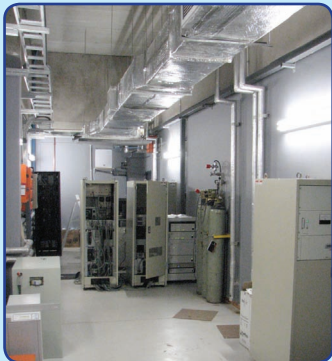
Images of the user rooms, housing the noisy auxiliary equipment for the microscopes. The services are fed through a trench in the floor. These are at the back of the microscope labs.
