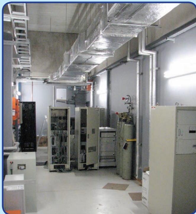
Images of the user rooms, housing the noisy auxiliary equipment for the microscopes. The services are fed through a trench in the floor. These are at the back of the microscope labs.
